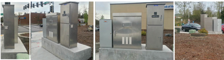
Example of standard utility box.
